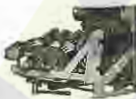
PLB in open position with fuses racked-out
