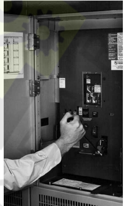
Two-Step Stored-Energy Closing
