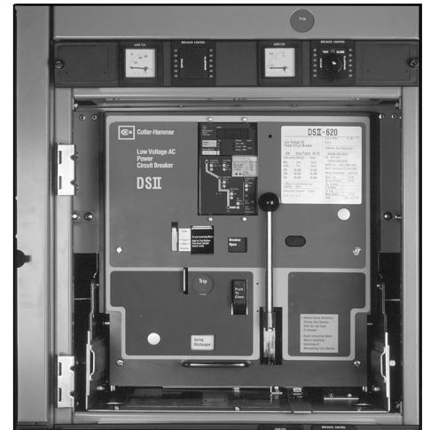
Cell With Breaker
